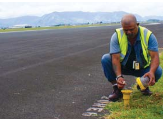
An international airport requires attention to thousands of details, all important in their own right - checking landing strip lighting is one.
